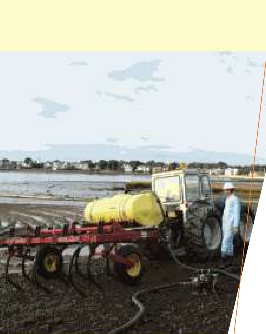
Filling Tank on Oxidant Delive
